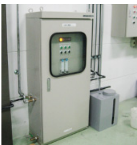
Full automatic Airkem spraying unit
